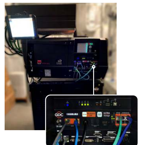
Projector in K11 Art House uses GDC SR-1000 media server
